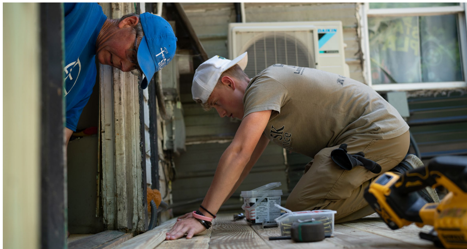
Lee Martin, an Appalachia Build staff member, and volunteer Isaiah Turley construct a wheelchair ramp on a home in Kimball, West Virginia. Above, Carol Dunn makes lunch for volunteers in the kitchen of Houston United Methodist Church in Kimball.
