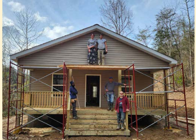
Inkosiinhle Ndlovu-Mathuthu (Zimbabwe), from left, finishes siding a house with other Mennonite Disaster Service volunteers in Eastern Kentucky including Angela and Daryl Stauffer, Chris Rhodes and Carl Ranck.
