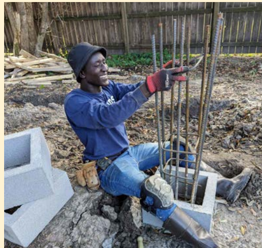
Jack Odhiambo (Kenya) works to apply stirrups to the rebar for the footers on a new house in Jennings, Louisiana, during his assignment with Mennonite Disaster Service.
