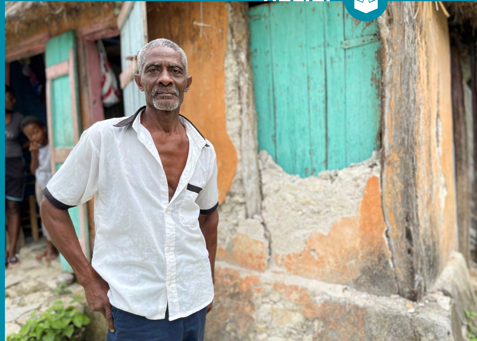
Pierre Hérorol stands in front of his badly damaged home that he shares with five other people. He received emergency food and supplies distributed by an MCC partner in Saint-Jean-du-Sud, Haiti, after the August 2021 earthquake. (MCC photo/Paul Shetler Fast)
